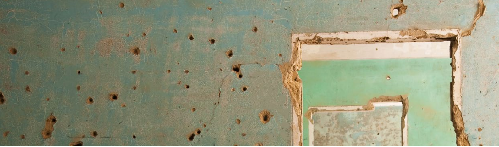
Interior of the abandoned and bullet-scarred hospital in Quneitra, Syria. iStock.com / Joel Carillet
